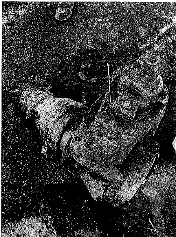
Existing failed water valve
