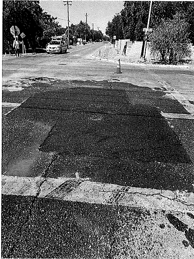
New valve cross pavement @ Q Street
